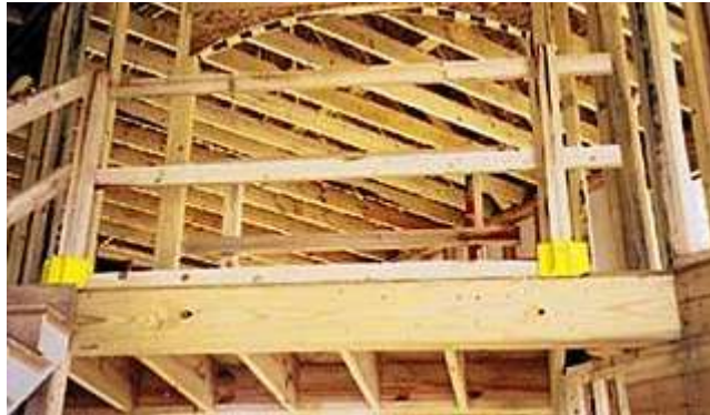
Figure 34 - A landing protected by a wooden guardrail system with a toeboard.
