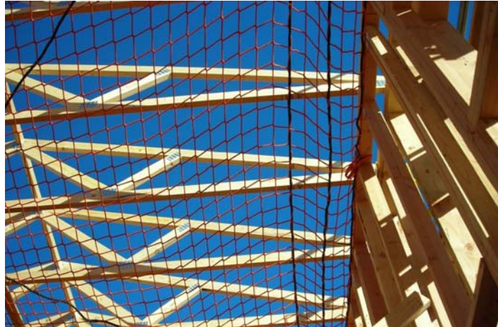
Figure 7 - An example of a safety net system.
