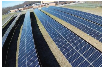
Solar arrays at Neimann elementary school.
