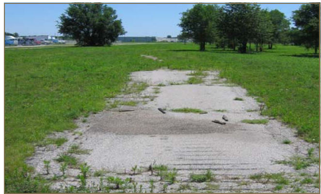
Areas of concrete remain at the site from its operations as a rail-road switch yard.
