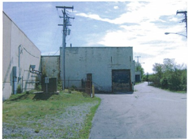
Photo 28: Viewing Pool and slab-mounted transformers at southwest corner of main
