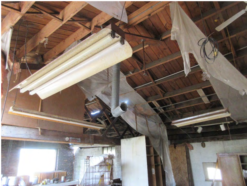
Photograph No. 7: Fluorescent light ballasts (4-foot and 8-foot) inside North Building. Possible PCB transformers and mercury vapor light bulbs.
