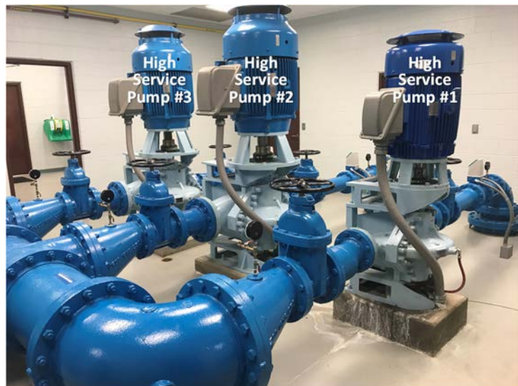
Figure 15. Existing high service pumps
