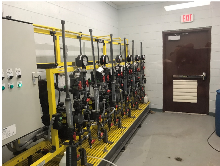
Figure 22. Existing chlorine feed system
