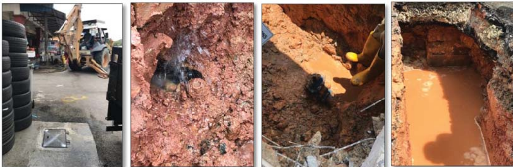
Figure 17.18.3 Excavations and leaks. (Source: Primayer)
