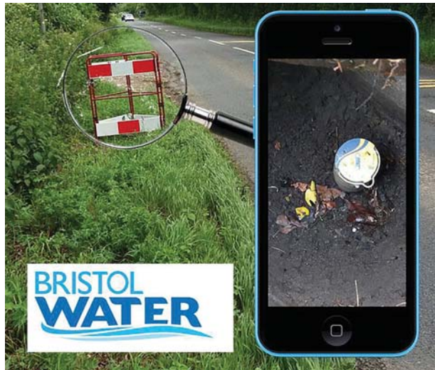
Figure 17.11.1 Enigma installation next to the A4135 highway. (Source: Primayer)
