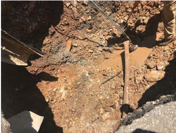
Figure 17.14.2 Excavated leak (Source: Xylem)
