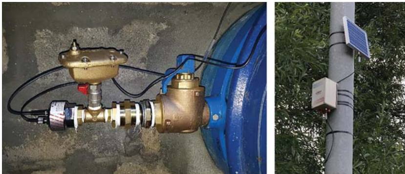
Figure 9.2 Solar-powered 3G data gateway on a nearby pole (right) and hydrophone sensor with external antenna and battery pack, plus automatic bleeding valve (left). (Source: Gutermann)
