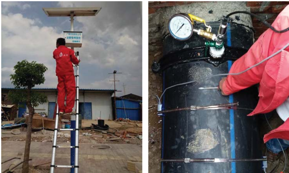
Figure 17.9.3 Field work of metering devices installation and calibration. (Source: Yunnan Kan Zheng Water Loss Control & Engineering Co., Ltd)
