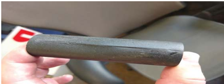
Figure 17.14.3 A longitudinal split on one of the seven leaking HDPE service lines that were buried deep below the surface. (Source: Xylem)
