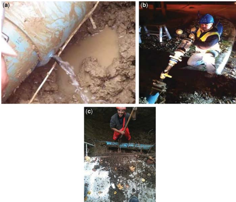
Figure 17.8.1 (a) and (b) Leak located on MDPE electro-fusion joint, (c) located joint on MDPE pipe where leak detected. (Source: JD7 Ltd)
