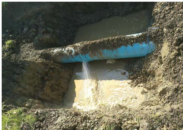
Figure 17.17.4 Detected leak. (Source: Primayer)
