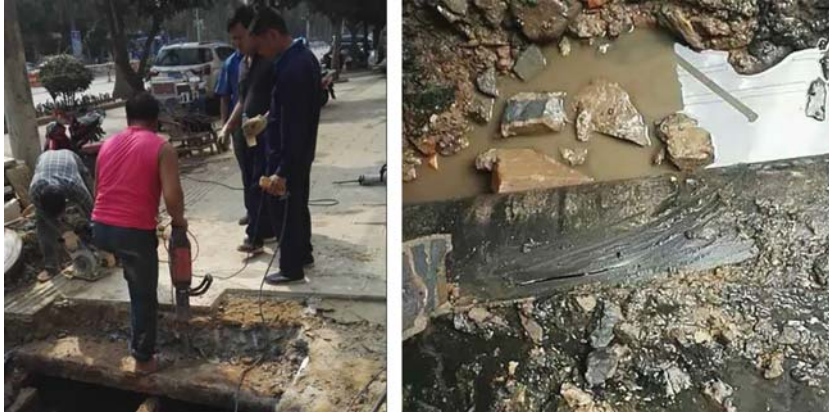
Figure 17.9.8 Leak point confirmation. (Source: Yunnan Kan Zheng Water Loss Control & Engineering Co., Ltd)
