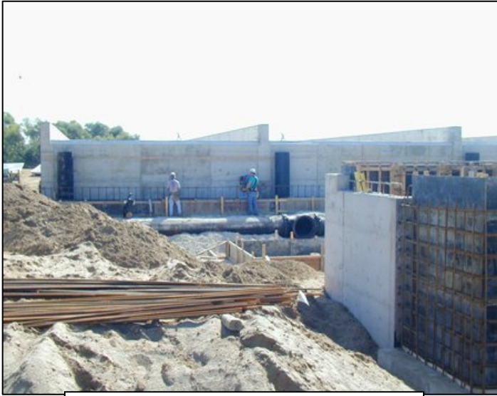
Sullivan's new CSO storage facility.
