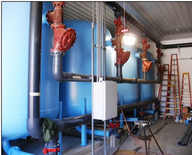
Brookston's new pressure filtration units.
