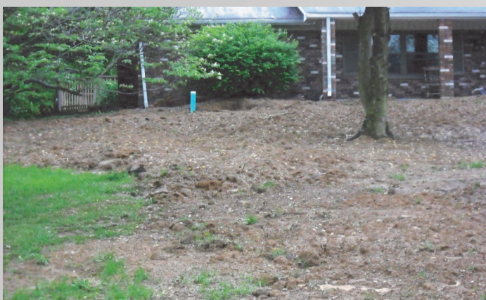
One of houses along Stonehaven Circle that has been connected to sewer system.
