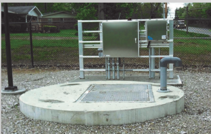
Stonehaven main lift station constructed on SR #61.
