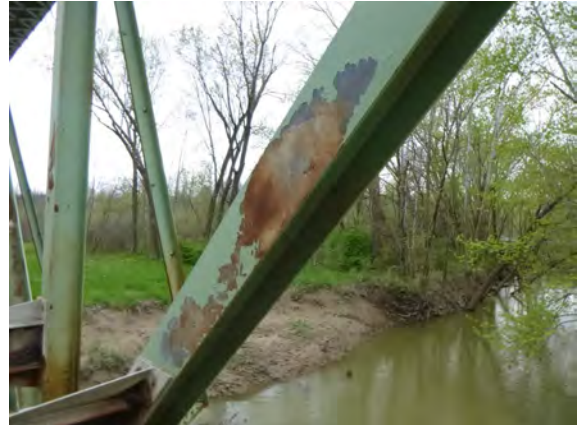
L4U3 NORTHWEST PAINT PEELING
