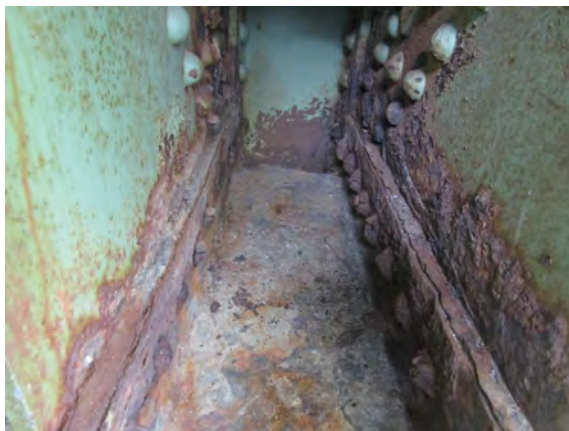
EXPANSION RUST AND SECTION LOSS AT NEL0
