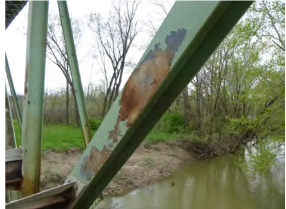
L4U3 NORTHWEST PAINT PEELING
