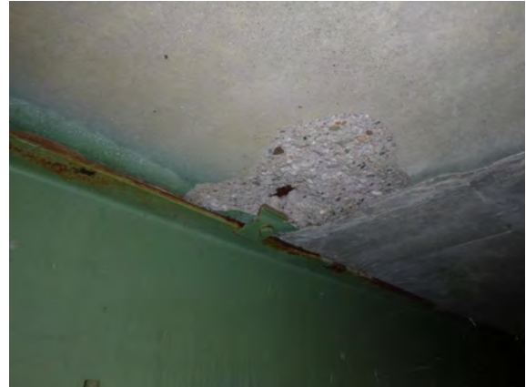
SPALL WITH EXPOSED REINFORCEMENT IN DECK
