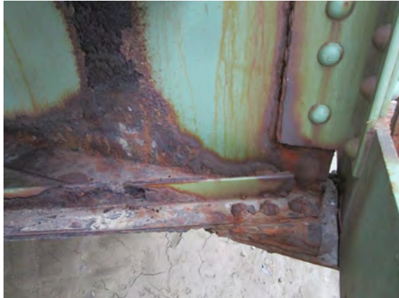
TYPICAL FLOOR BEAM DETERIORATION AT BOTTOM FLANGE
