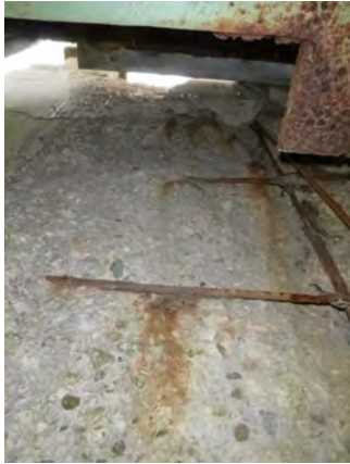
NORTHWEST ABUTMENT 2 SPALL IN MUDWALL
