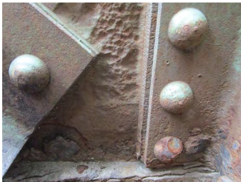
PHOTO 36: SEL2L1 INTERIOR GUSSET PLATE SECTION LOSS AT DIAGONAL END
