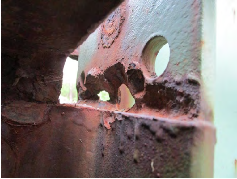
PHOTO 40: NEL1 60% SECTION LOSS ON INTERNAL FLANGE OF VERTICAL
