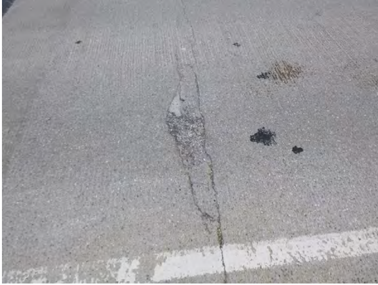
PHOTO 22: OVERLAY SPALL NORTH END
