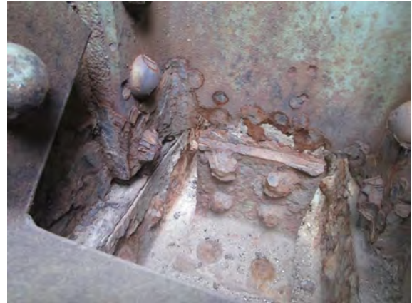
EL4 WEB CONNECTION SEVERED FROM LOW CHORD
