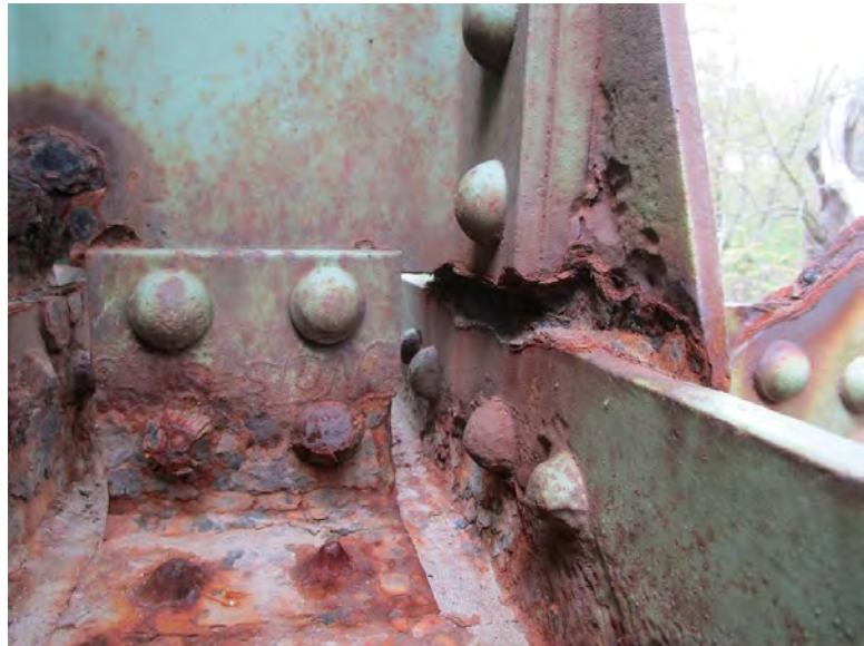
PHOTO 35: SEL1 EXTERIOR GUSSET PLATE SECTION LOSS
