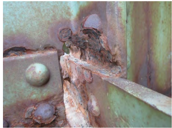
SEL1 INTERIOR ANGLE SECTION LOSS
