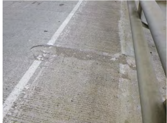
OVERLAY SPALL MIDSPAN WEST COPING
