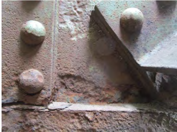
SEL2L1 EXTERIOR GUSSET PLATE SECTION LOSS AT DIAGONAL END
