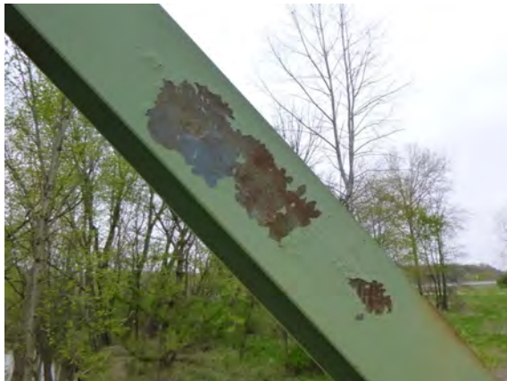
L2U3 NORTHWEST PAINT PEELING
