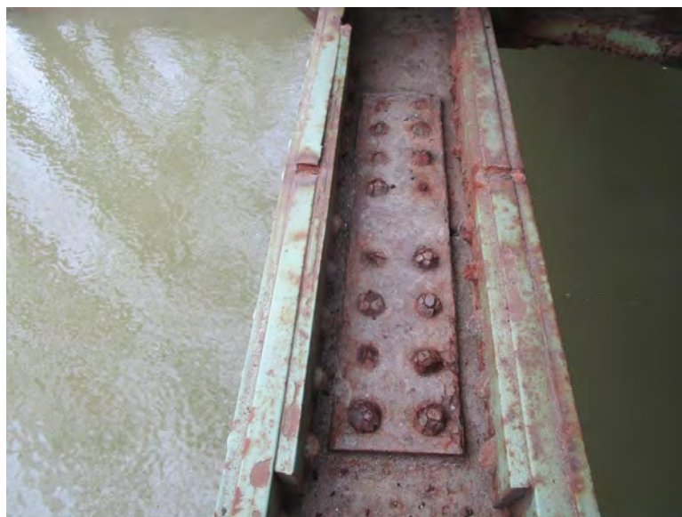
PHOTO 39: TYPICAL LOW CHORD SPLICE
