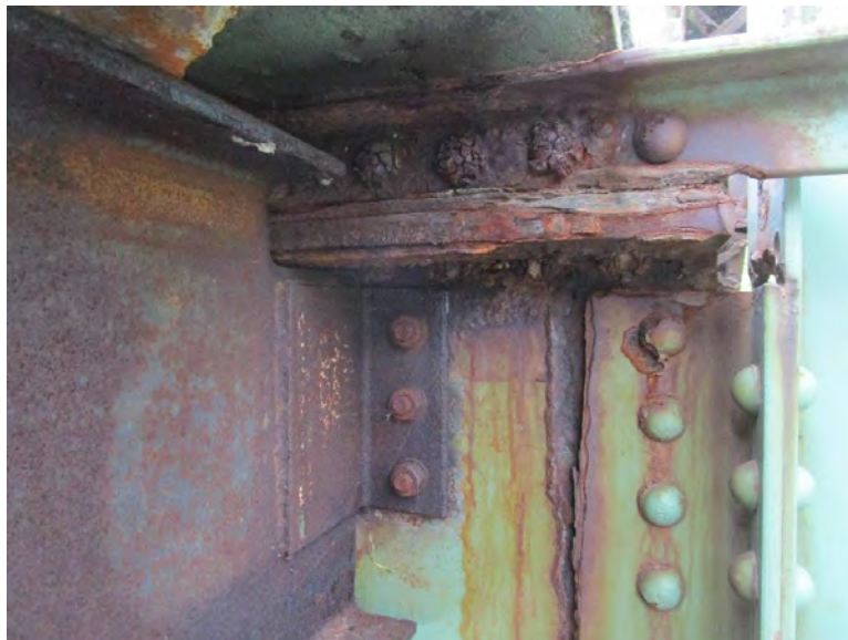
PHOTO 42: TYPICAL FLOOR BEAM DETERIORATION AT TOP FLANGE
