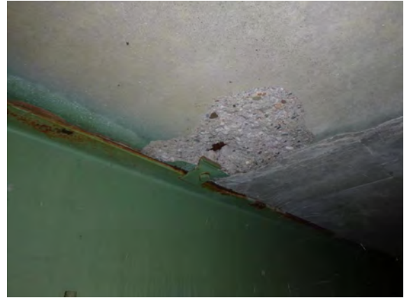
SPALL WITH EXPOSED REINFORCEMENT IN DECK
