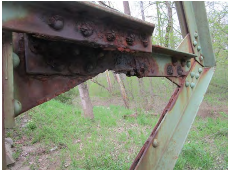
PHOTO 41: TYPICAL DETERIORATION OF EXTERNAL SWAY BRACING
