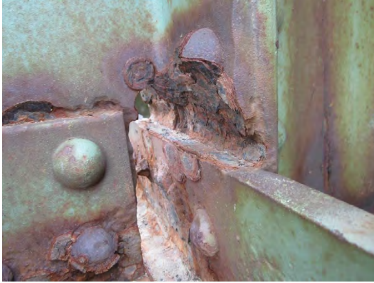
PHOTO 34: SEL1 INTERIOR ANGLE SECTION LOSS
