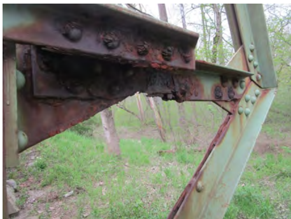
TYPICAL DETERIORATION OF EXTERNAL SWAY BRACING
