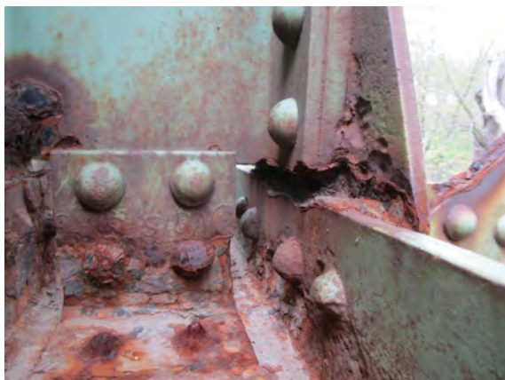
SEL1 EXTERIOR GUSSET PLATE SECTION LOSS
