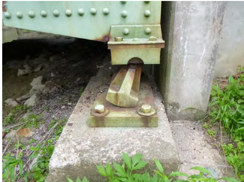
PHOTO 29: OVER ROTATED EXPANSION BEARING
