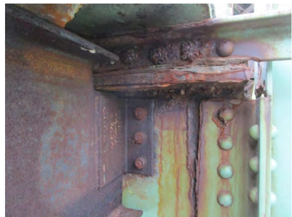
TYPICAL FLOOR BEAM DETERIORATION AT TOP FLANGE
