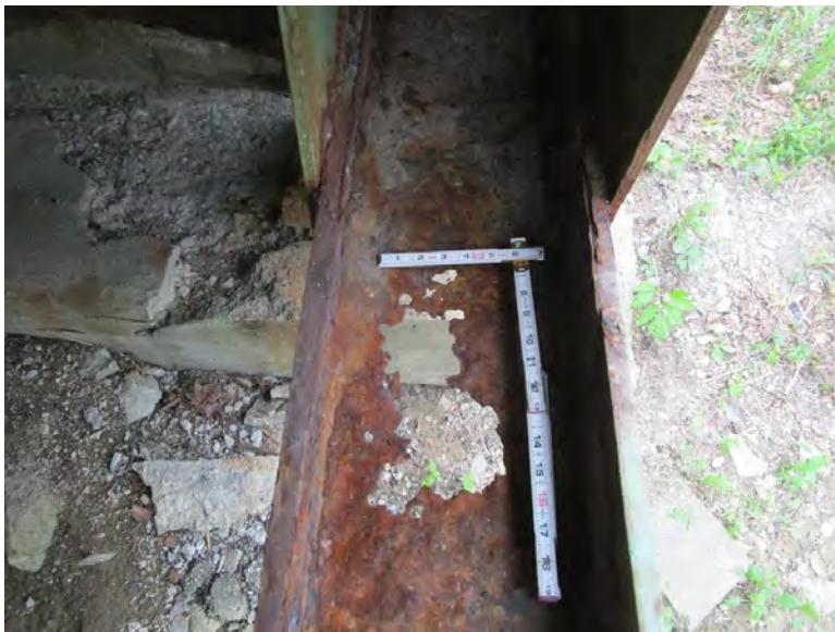
PHOTO 30: MODERATE SECTION LOSS IN WEB AT NELO
