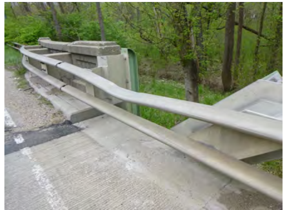
DAMAGED EAST GUARDRAIL
