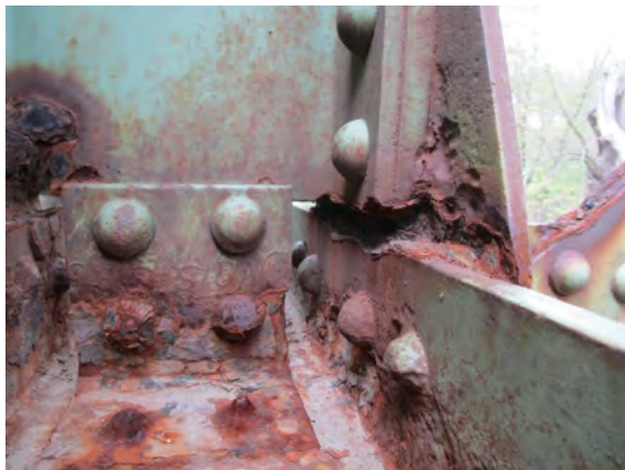
SEL1 EXTERIOR GUSSET PLATE SECTION LOSS
