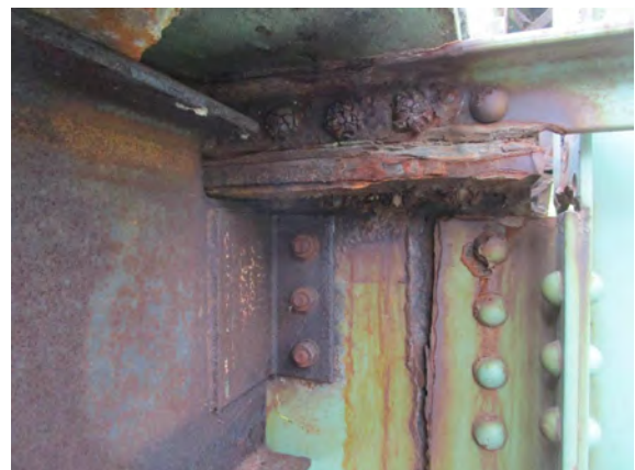
TYPICAL FLOOR BEAM DETERIORATION AT TOP FLANGE
