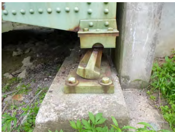
OVER ROTATED EXPANSION BEARING
