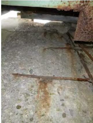
NORTHWEST ABUTMENT 2 SPALL IN MUDWALL
