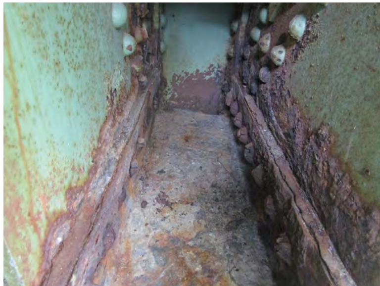
PHOTO 33: EXPANSION RUST AND SECTION LOSS AT NELO
