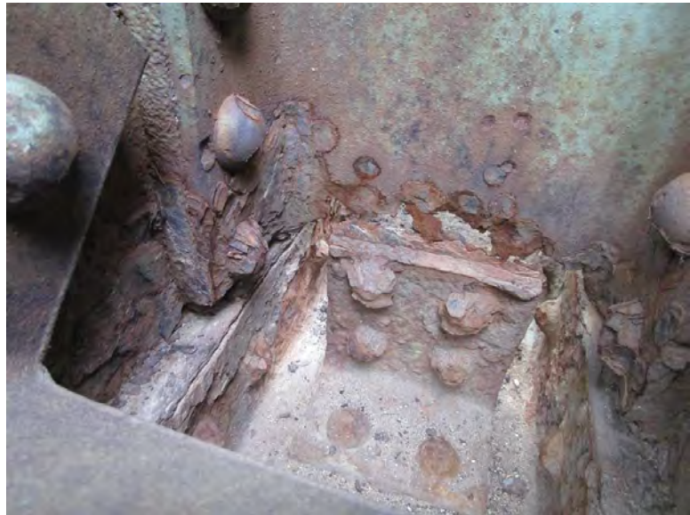
PHOTO 38: EL4 WEB CONNECTION SEVERED FROM LOW CHORD
