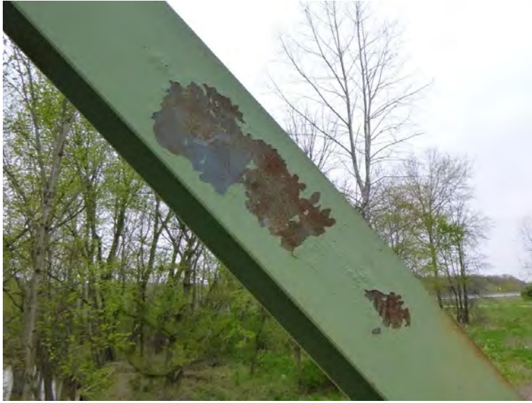
PHOTO 28: L2U3 NORTHWEST PAINT PEELING
