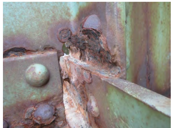
SEL1 INTERIOR ANGLE SECTION LOSS
