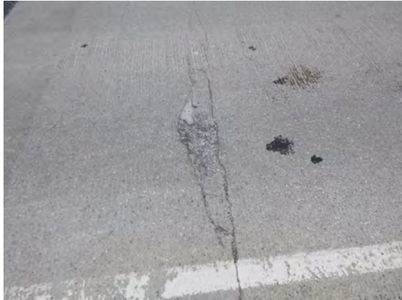
OVERLAY SPALL NORTH END
