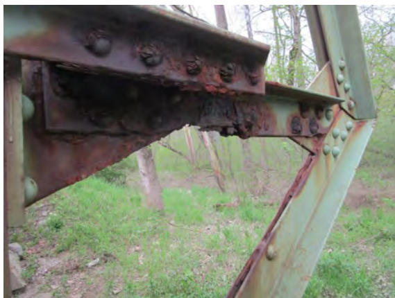
TYPICAL DETERIORATION OF EXTERNAL SWAY BRACING
