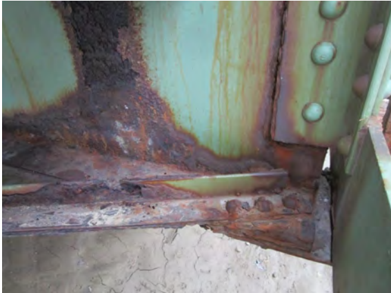
TYPICAL FLOOR BEAM DETERIORATION AT BOTTOM FLANGE
