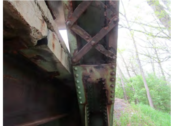
TYPICAL HEAVY SECTION LOSS OF STAY PLATES AND LATTICE BARS ON END POST
