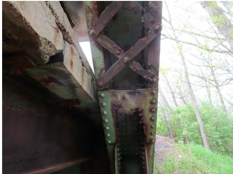
PHOTO 44: TYPICAL HEAVY SECTION LOSS OF STAY PLATES AND LATTICE BARS ON END POST
