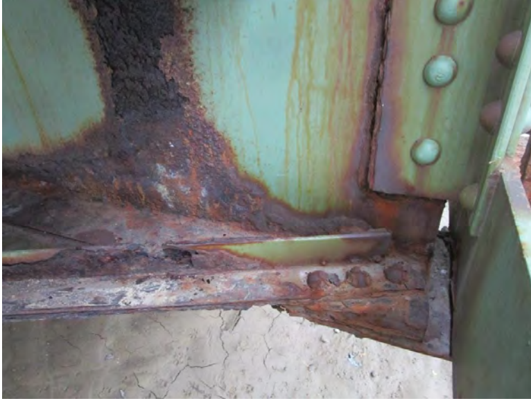
PHOTO 43: TYPICAL FLOOR BEAM DETERIORATION AT BOTTOM FLANGE
