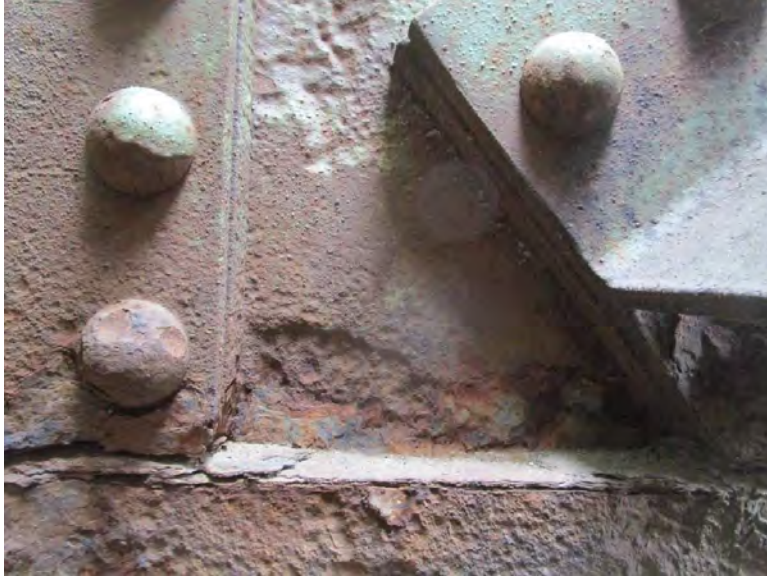
PHOTO 37: SEL2L1 EXTERIOR GUSSET PLATE SECTION LOSS AT DIAGONAL END
