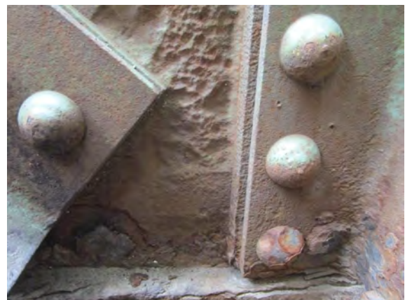
SEL2L1 INTERIOR GUSSET PLATE SECTION LOSS AT DIAGONAL END
