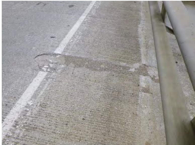
PHOTO 23: OVERLAY SPALL MIDSPAN WEST COPING
