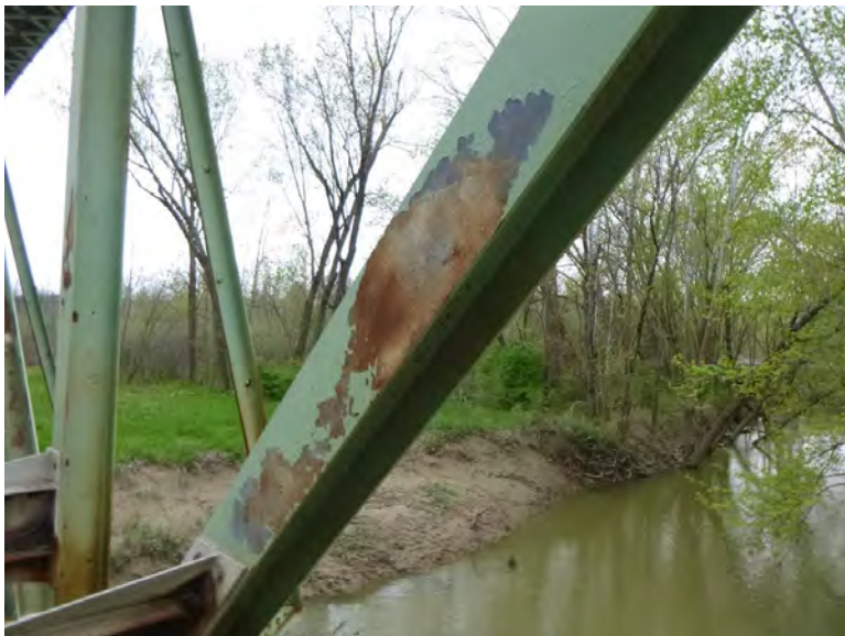
PHOTO 27: L4U3 NORTHWEST PAINT PEELING
