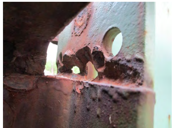
NEL1 60% SECTION LOSS ON INTERNAL FLANGE OF VERTICAL
