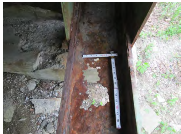
MODERATE SECTION LOSS IN WEB AT NEL0
