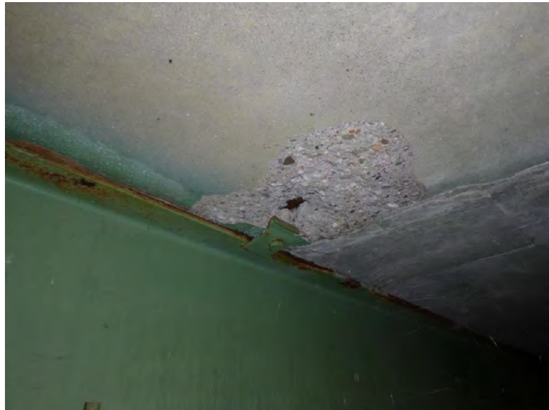
PHOTO 32: SPALL WITH EXPOSED REINFORCEMENT IN DECK
