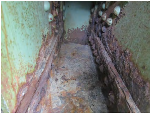
EXPANSION RUST AND SECTION LOSS AT NEL0
