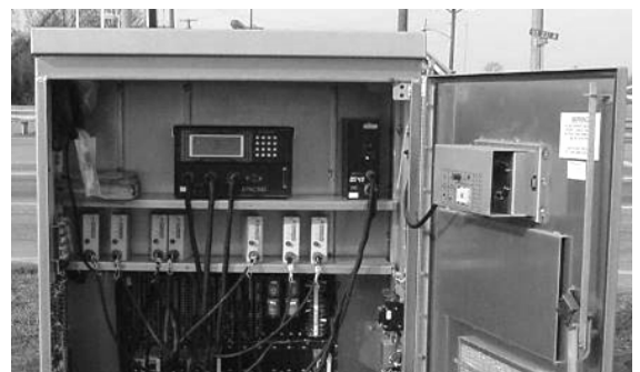
Figure 1-9 Controller Cabinet Wiring
