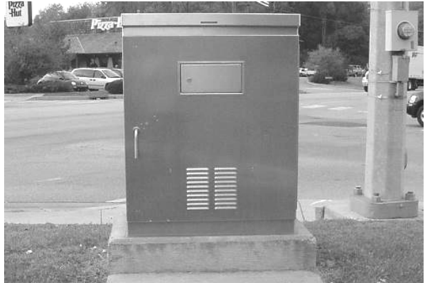
Figure 1-8 Traffic Signal Controller
