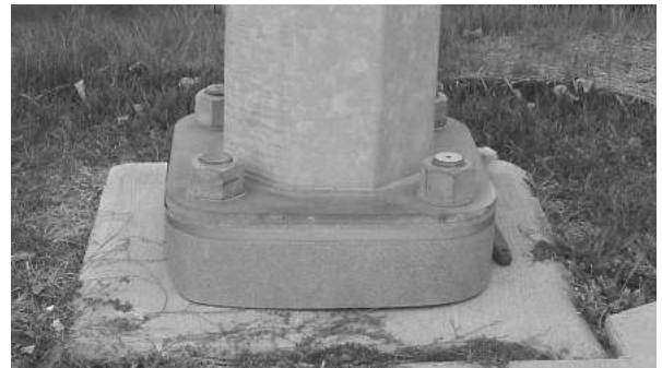
Figure 1-1 Steel Strain Pole
