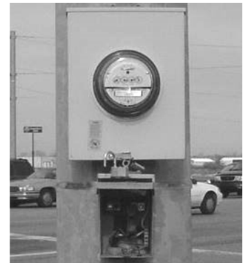
Figure 1-7 Electrical Service and Entrance Switch
