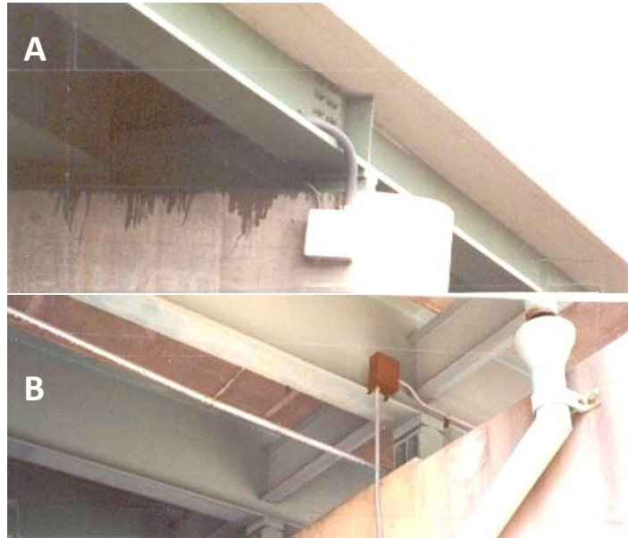
Figure 4-2 Errors in Underpass Breaker Box Installation (a) Top entry is not allowed (b) 2" conduit not attached at 4' intervals
