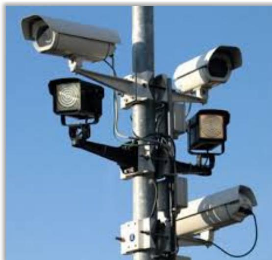
Figure 3-4: Traffic Camera Array (NTTA)
