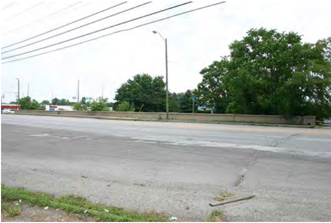
7_Looking NE at teh railing of the SE section of Bridge 2410F
