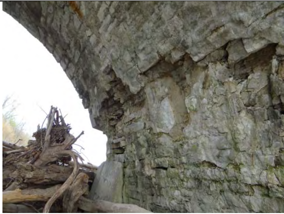
Figure 2 - 2012 - looking at Pier 3 west face - note voids and missing stones
