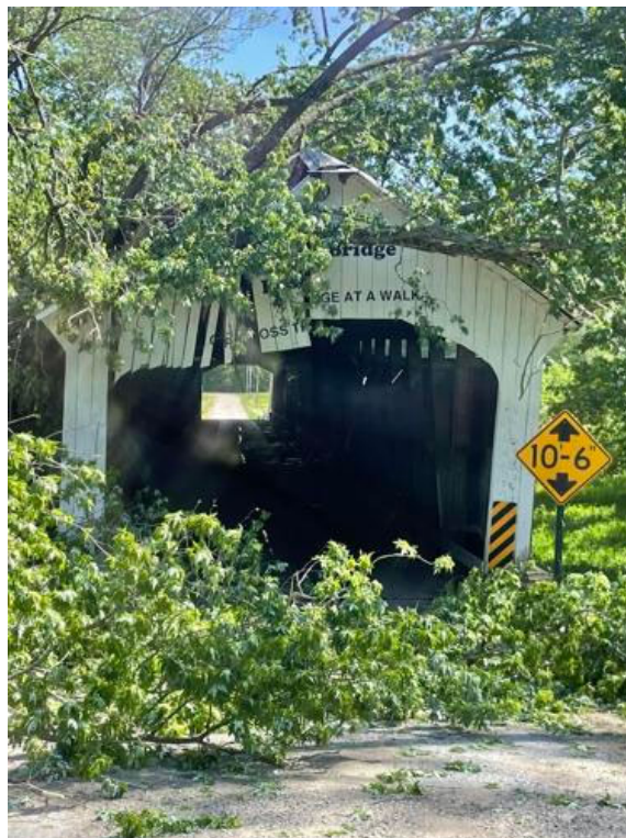
A tree has fallen on the Roseville Covered Bridge in Parke County. Submitted photo
