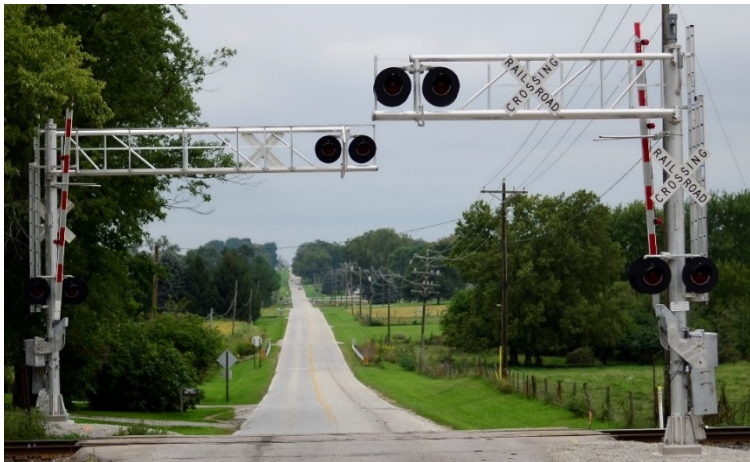
Figure 2-24 – Typical Section 130 Program Project: New Train-Activated Flashing Light Signals, Bell, Gates, Overhead Cantilever, Constant Warning Time Circuitry
