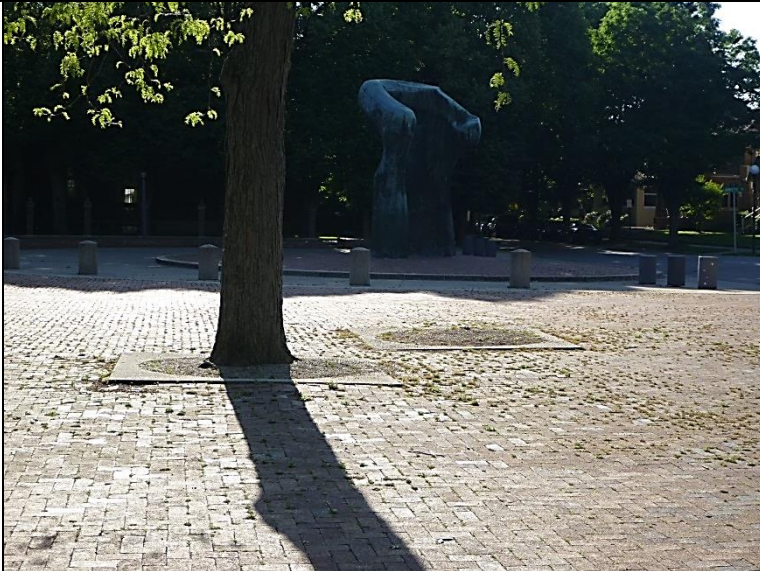
Before photo of main plaza showing uneven settling and deterioration of brick pavers
