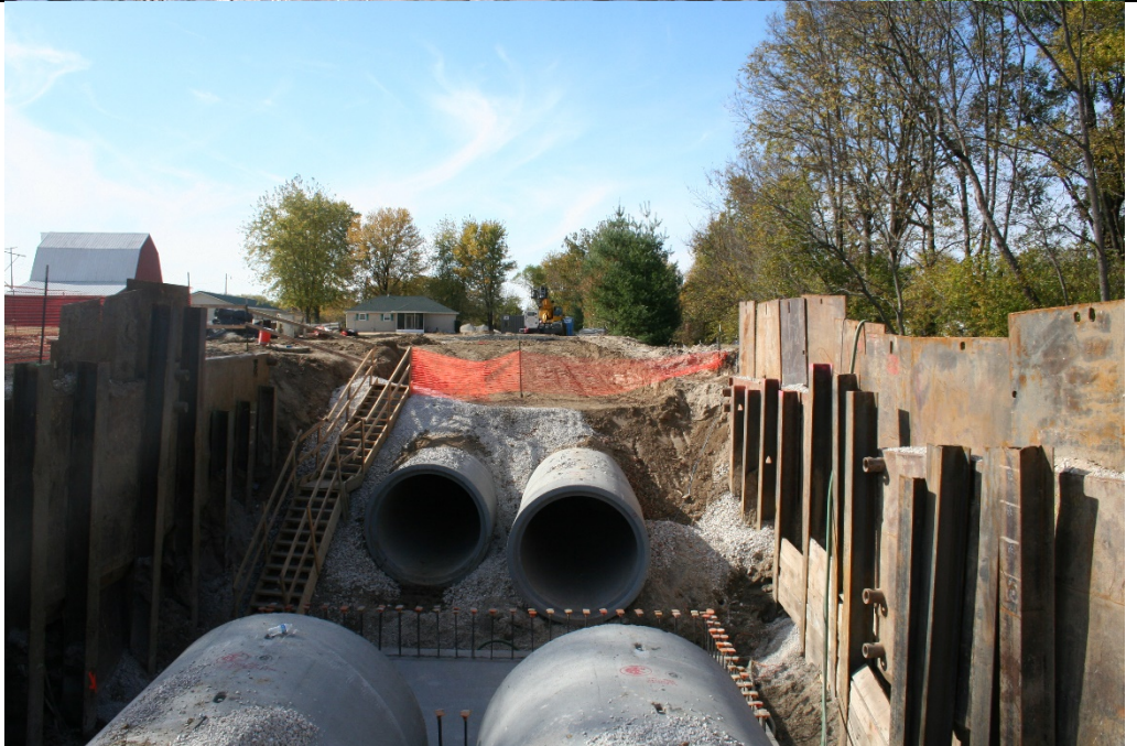
84-inch Conveyance pipes to the constructed wetland
