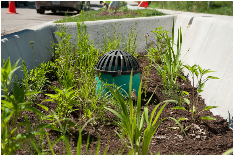
Overflow structure with domed grate
