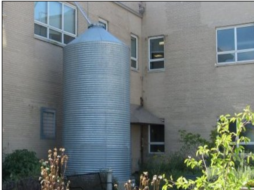
Figure 1 Above ground cistern, Chicago, IL (USEPA, picasaweb)
