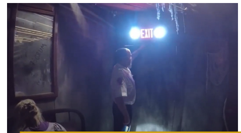
IDHS Code Enforcement Section field inspectors checking emergency exits in a haunted house.
